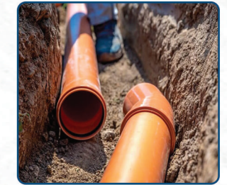
Strong Underground Drainage System
